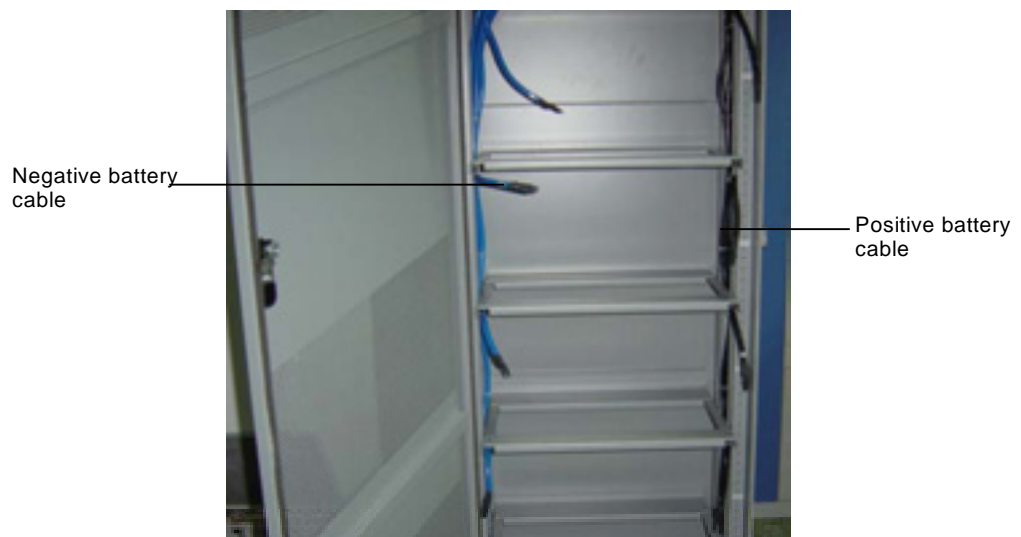
Figure 2-17 Positive and negative battery cables in each level
